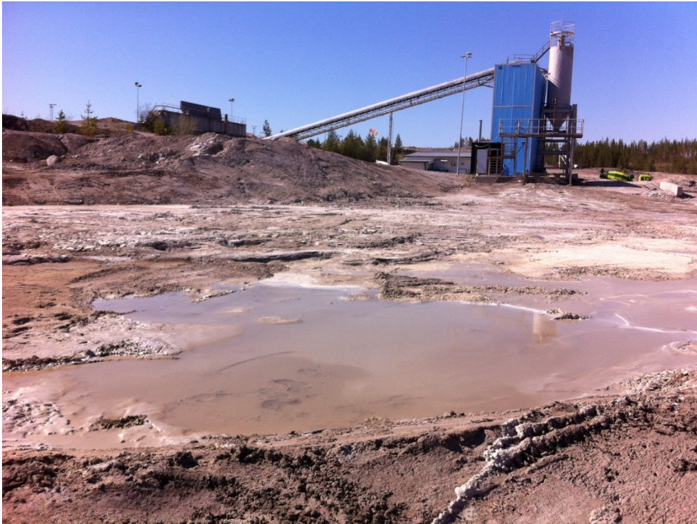
Figure 4. Sampling point at the wash pond at Skanska’s concrete plant, where the water from concrete lorries is collected after the lorries’ concrete tanks have been cleaned.
